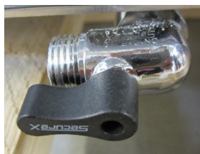
1. Control valve of steam generator
